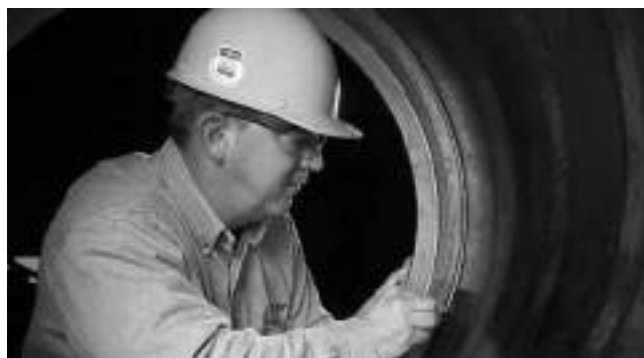
Fig. 238. Polishing out chock bore corrosion.
